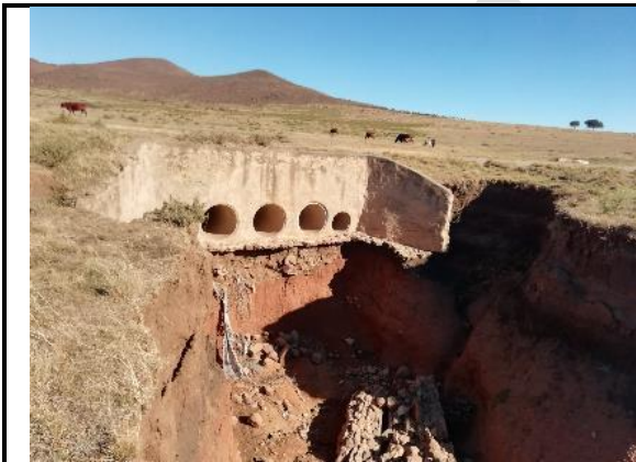
South western view of the pipe bridge over the tributary of the Mgwali River.
