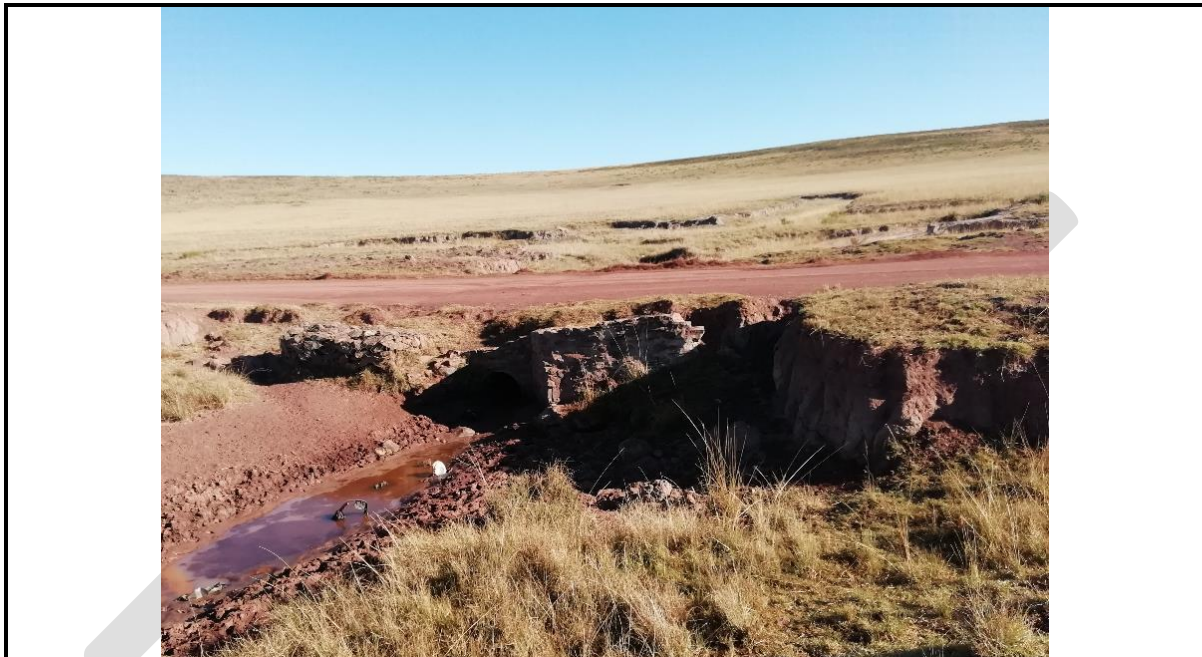
Existing pipe culvert structure over a tributary of the Kungxushungxushu River along the eastern section of the route upgrade.
