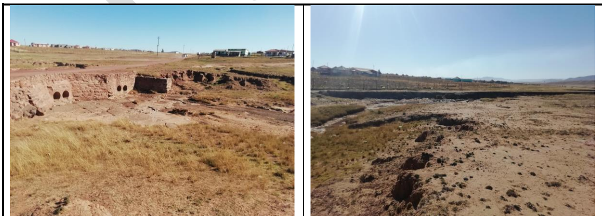
South western upstream view of the pipe bridge over a tributary of the Mgwali River.
