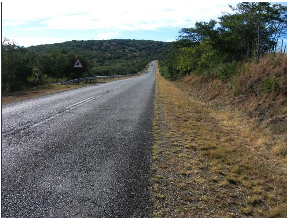
Fig. 3. View north-eastwards along the R63 (Section 16) to the east of the Gqunube River showing hilly terrain and low cuttings into weathered Beaufort Group bedrock (Loc. 303).
