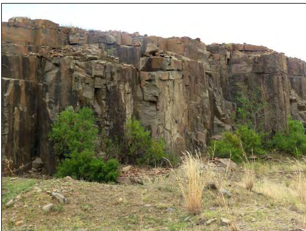
Figure 29. Cut face of existing quarry in the Q2 study area showing dolerite bedrocks with well-developed vertical sheet-like jointing.
