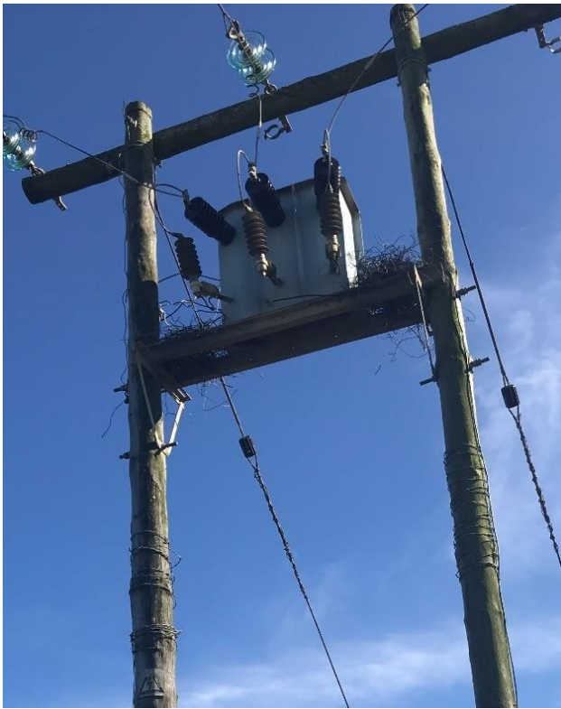
Figure 75: Crow nests constructed entirely out of wire may become a fire hazard.
