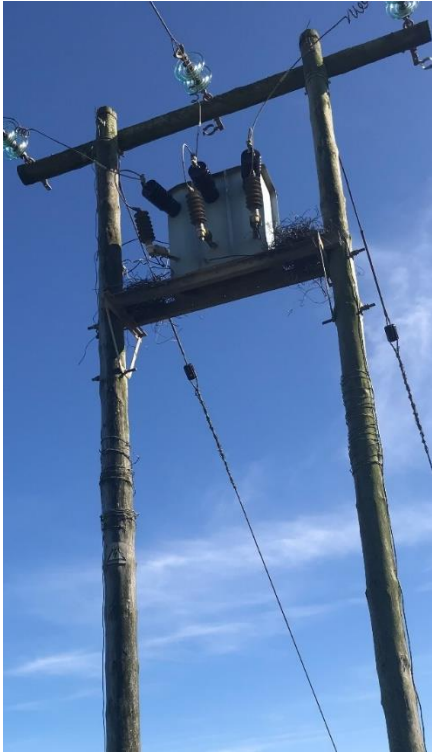
Figure 11: Crow nests constructed entirely out of wire may become a fire hazard.
